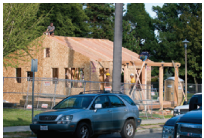
The pre-built home in its early stages, under construction at Alameda Park, before its move to Coyote Road.
